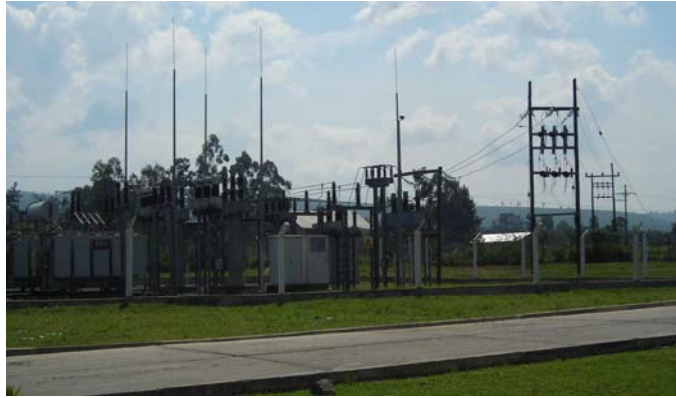
Electricity distribution infrastructure outside of Kisumu. Photo by author.
