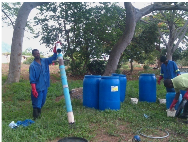
Photo by Moumié Maoulidi Pit Latrine
