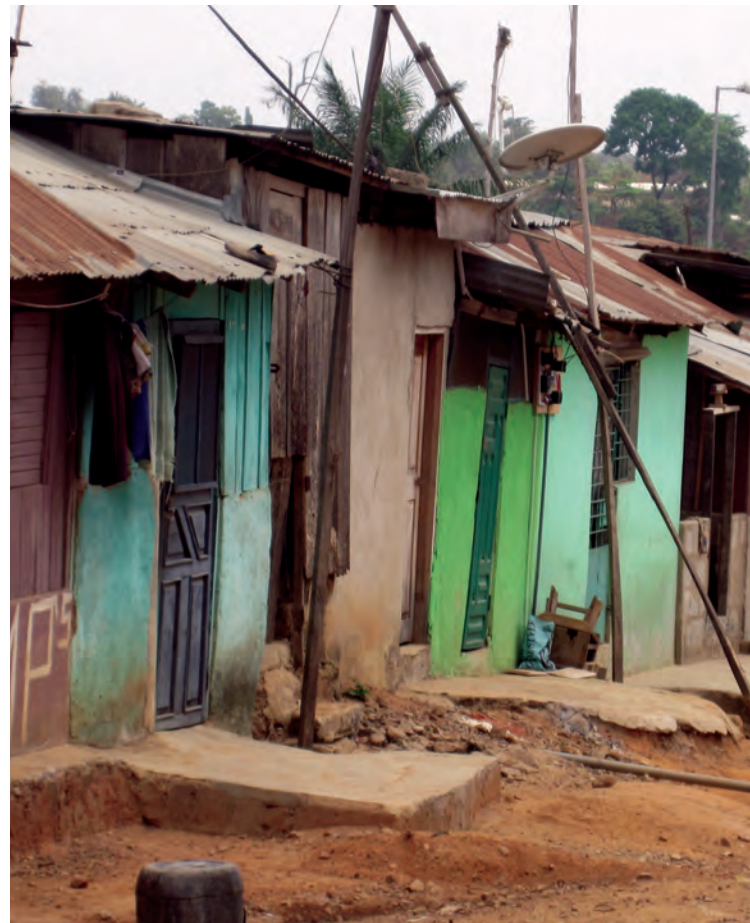
Many of the Millennium Cities, as depicted here in Accra, Ghana, suffer from overcrowding, driving residents into informal settlements with inadequate housing.
